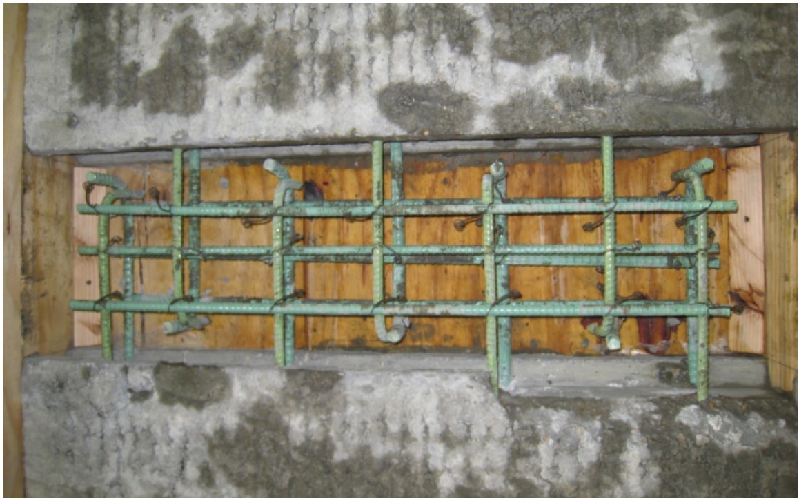
FIGURE 6-8: HOOKED BAR LAB PICTURES
